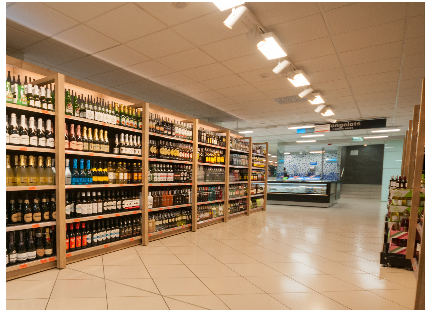
LUMINARIAS CARRIL TRACK FIXTURES
