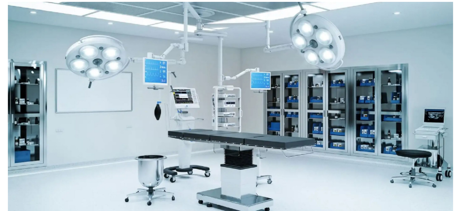
SALAS BLANCAS CLEAN ROOMS
